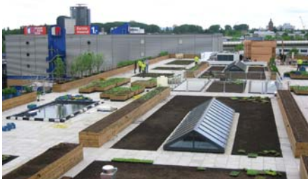
The system build-up "Sedum Carpet" with Fixodrain® XD 20 was applied between the skylights ...
